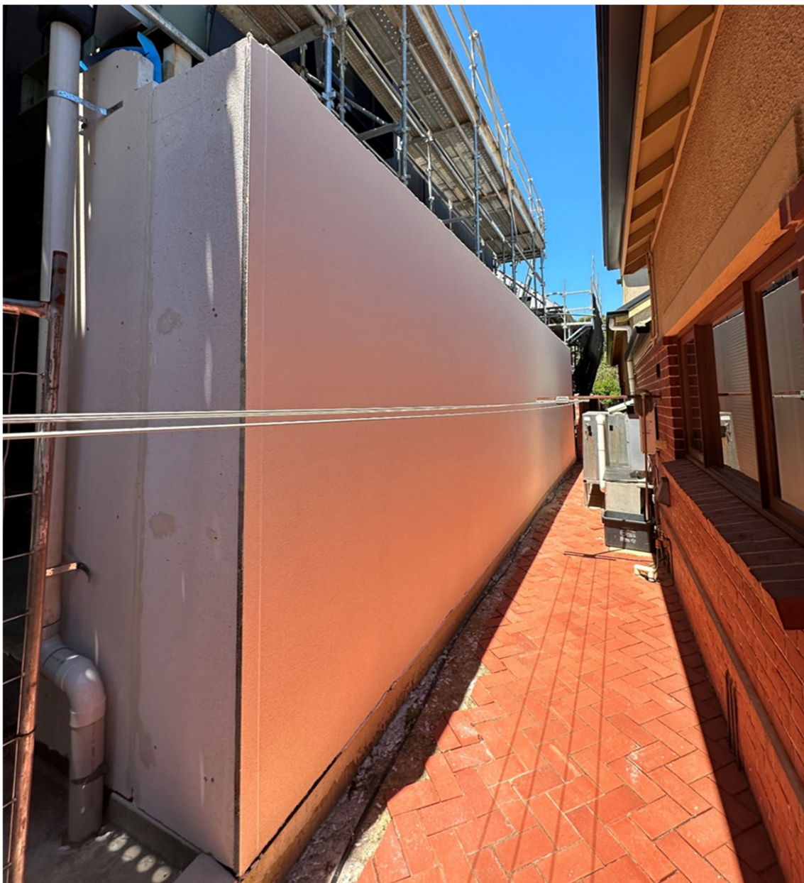
Image 1: Looking south-east, showing the proposed boundary wall (left) in relation to the adjacent dwelling (right).
