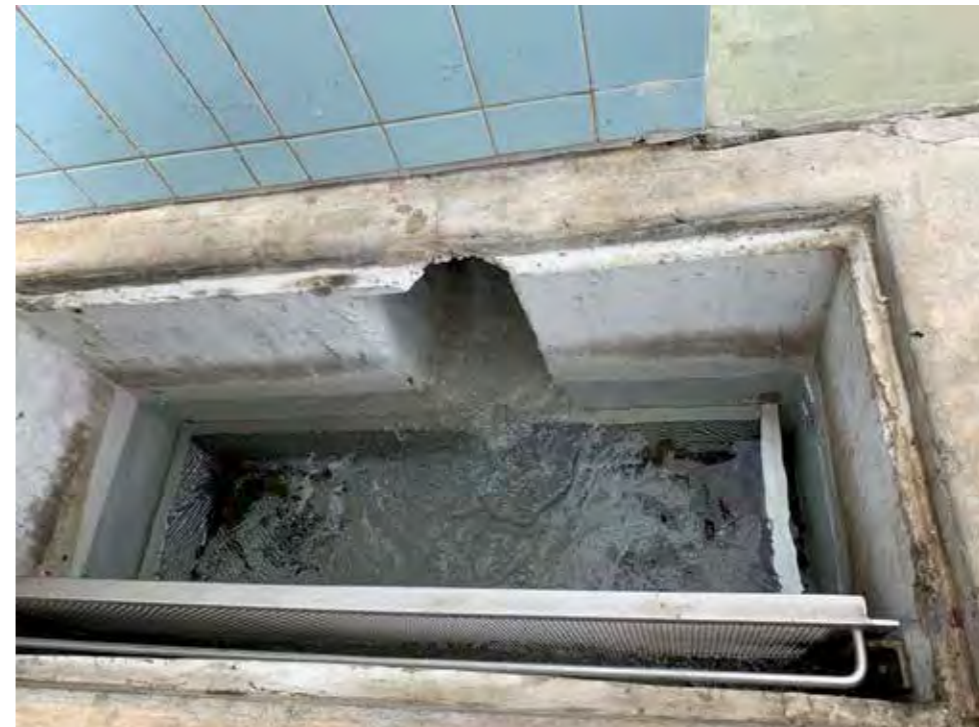
Figure 7: Scum gutter outlets at ends of channel
