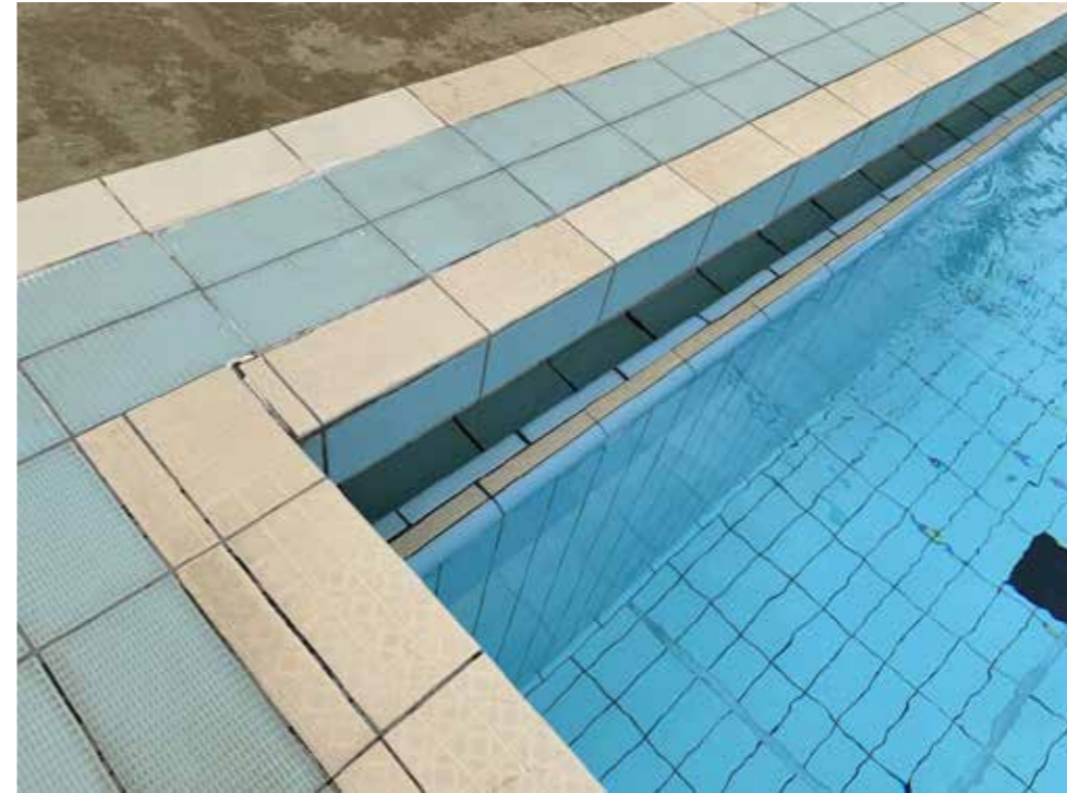
Figure 6: 50m Scum Gutter Removal system
