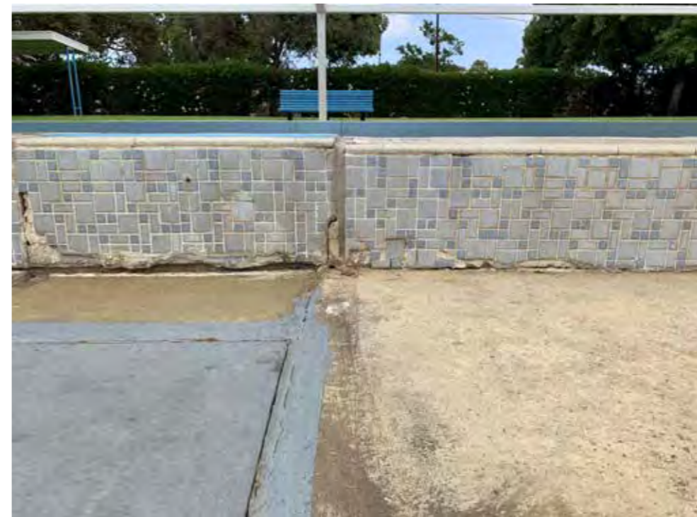
Figure 12: Movement in pool structure at central joint
