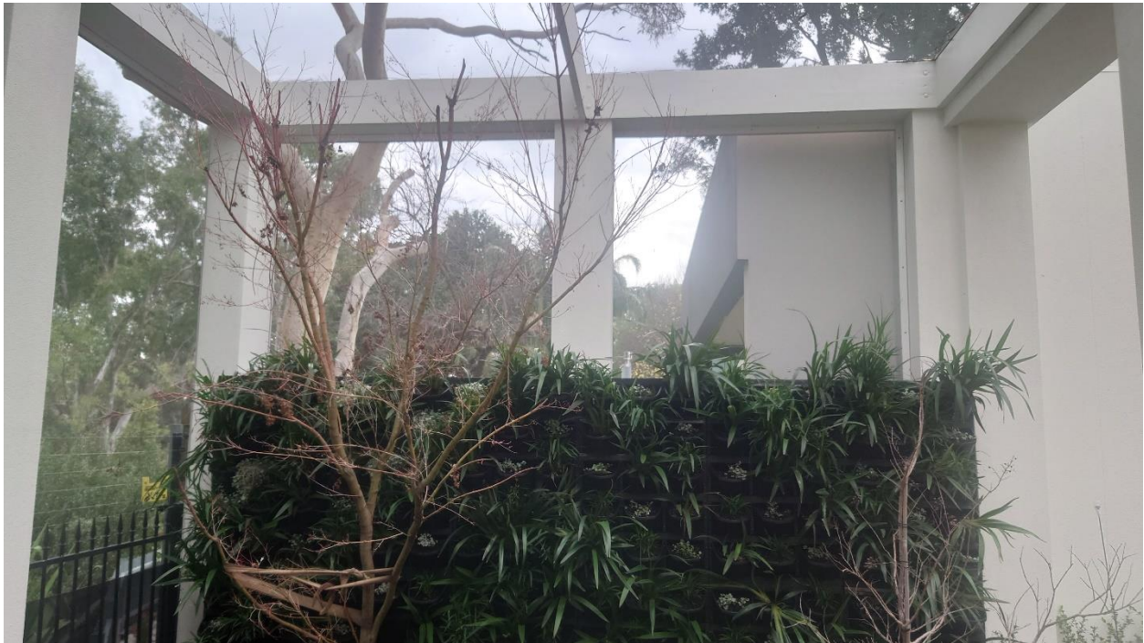
Image 3: View looking north of pergola structure with Neighbouring Boundary wall (44a) beyond (Source: Site Inspection Photo).
