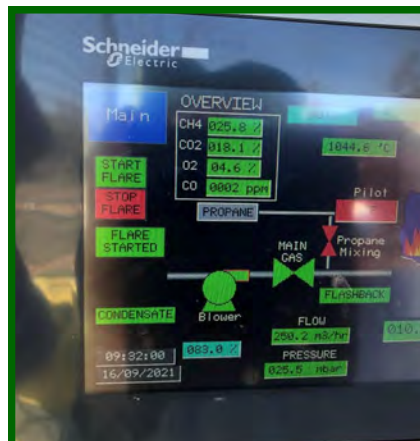
Control panel of flare operating
