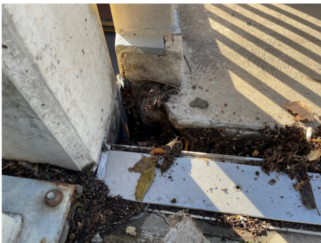
Figure 5 Pedestrian ramp concrete deterioration
