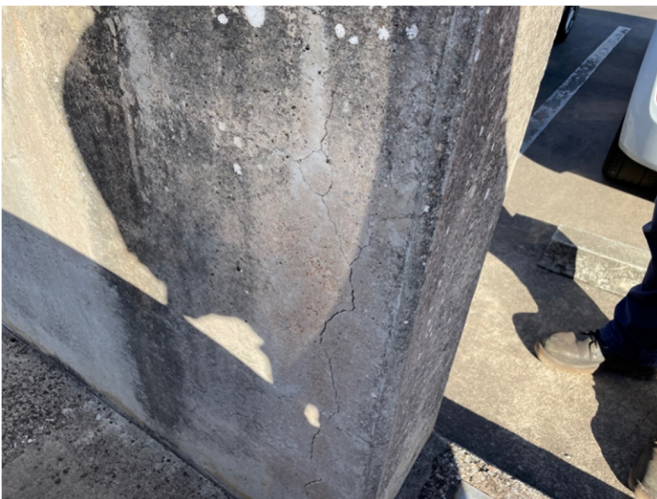
Figure 3 Spalling of top level column stubs
