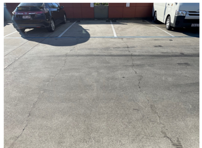
Figure 4 Top level slab cracking
