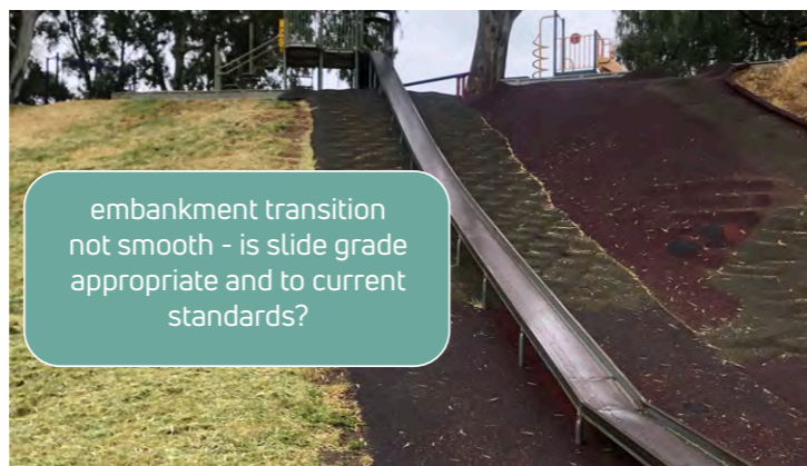
2. METAL EMBANKMENT SLIDE
